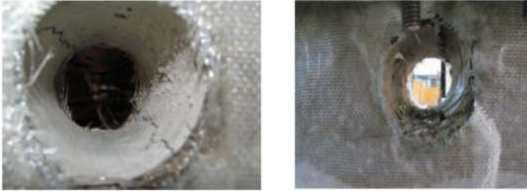
Fig.1 Cutout edges of FRP composite with threads loosened and the bond is weak between concrete and composite laminate [9]
